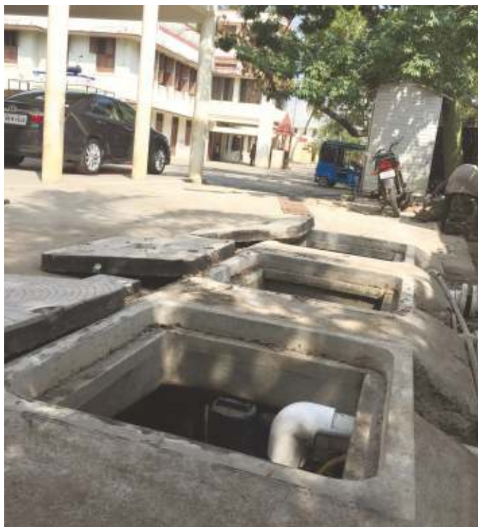
Sumps and pumps for stormwater
